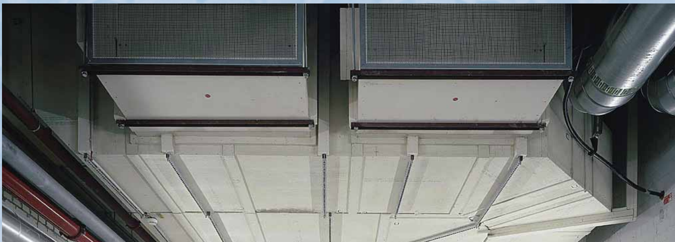
Vodorovné potrubí PROMATECT®-L500, E_{I_{multi}} 60
